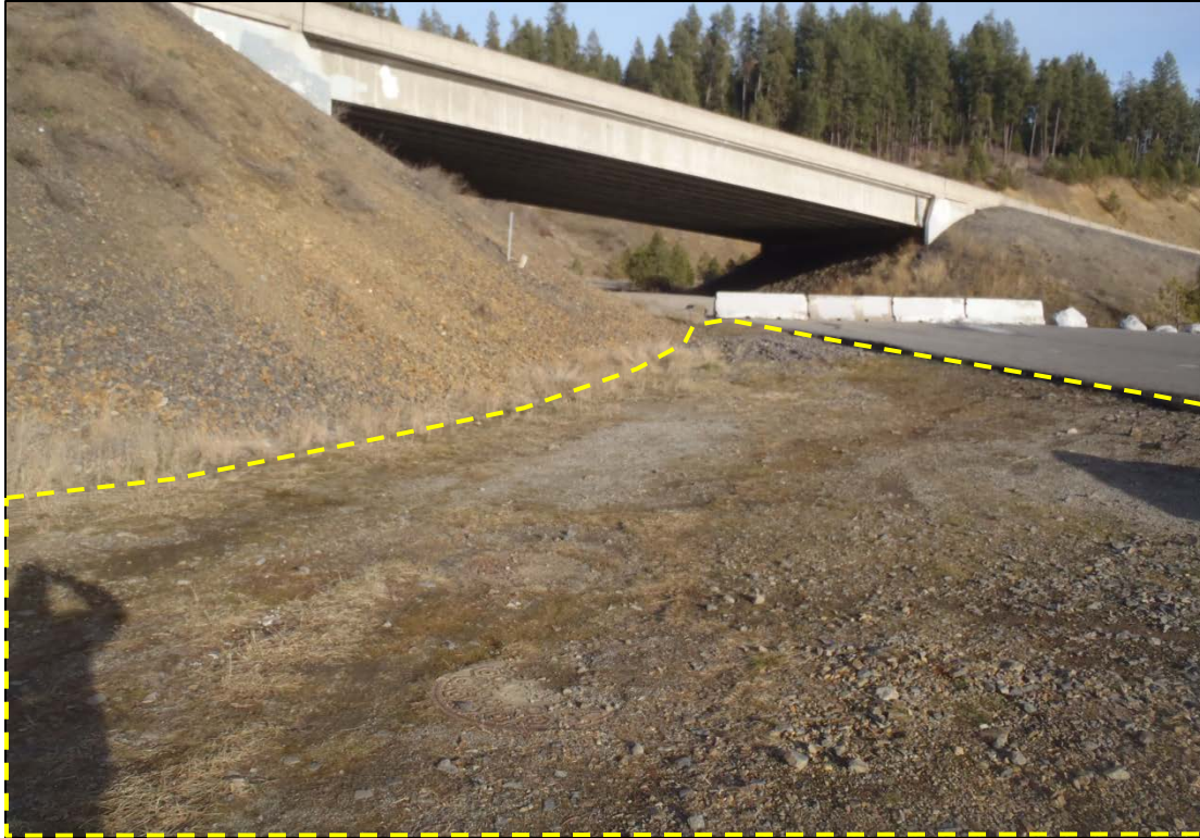
Photo 7. Looking east at unpaved right-of-way north of Coeur d'Alene Lake Drive/parking area for Higgens Point. The area outlined by the yellow dashed line will be raised to meet the grade of the asphalt to the right to allow the transport to turn under the overpass. The Jersey barriers blocking Coeur d'Alene Lake Drive would be temporarily removed during construction and transports. No public vehicular access is allowed past the barriers.
